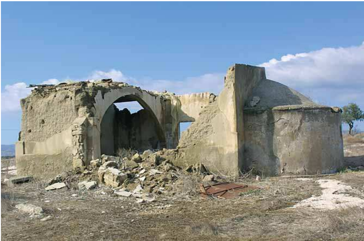
Archangel Michael's Church and cemetery in Trikomo after it was looted is now crumbling away.
