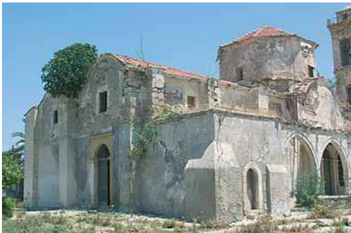
Cracks in the walls and the dome of the medieval church of the Archangel Michael in Lefkonoiko mark the danger of collapse.
