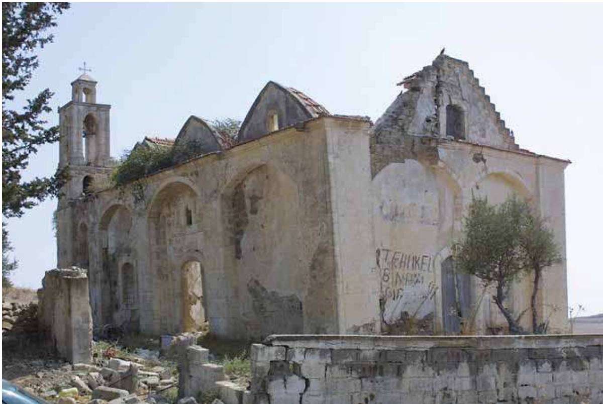
The St. George Church in Gerani after it was looted stands in a state of devastation and near collapse.
