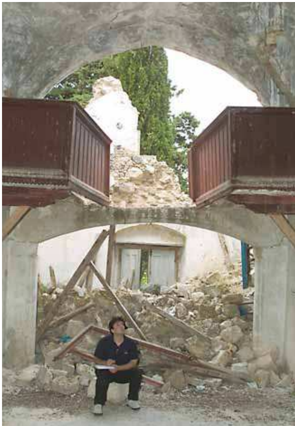
Part of Archangel Michael Church in Charkeia has completely collapsed.
