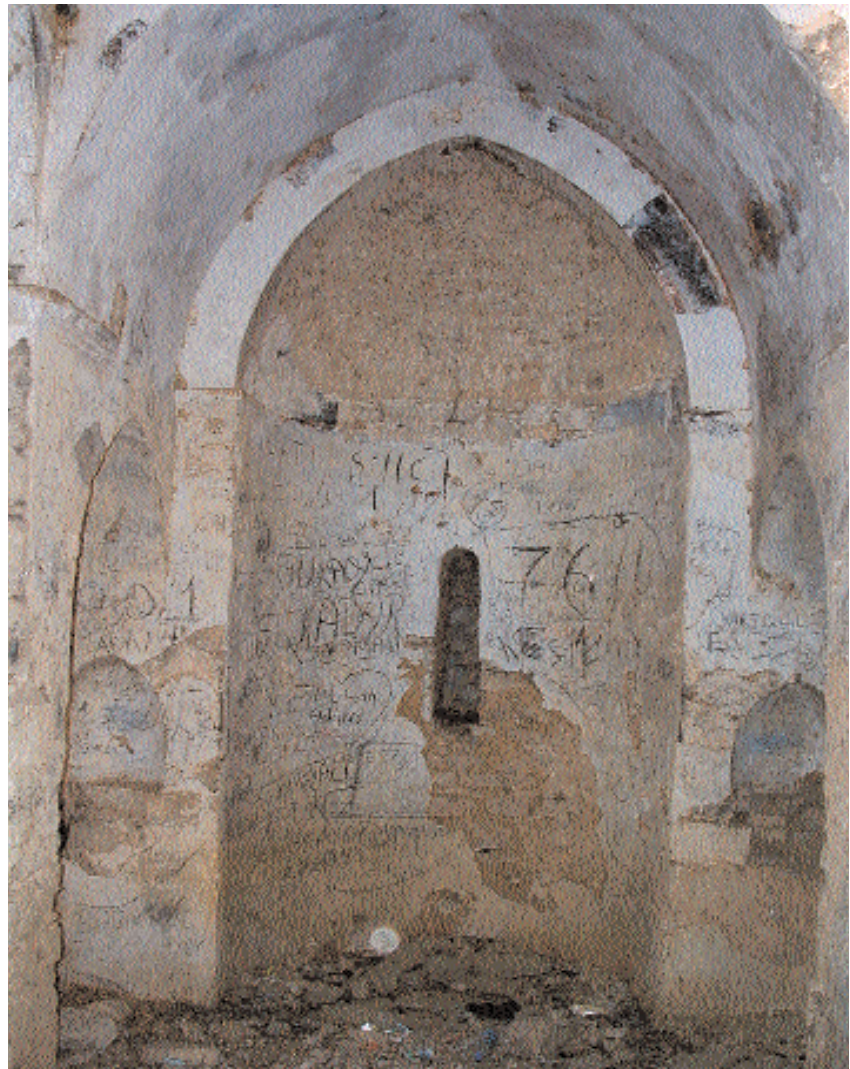
The present condition of the apse of the Hosios Euphemiaos church.
