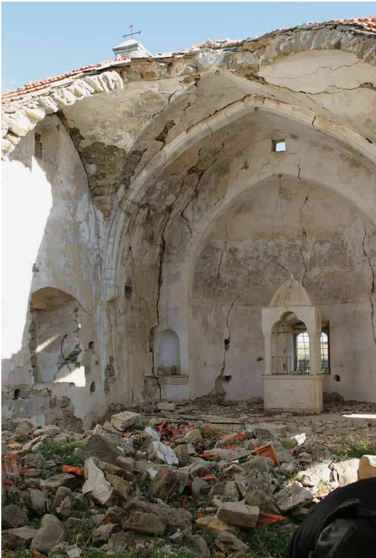
The collapse of the church of St. Georgios in Gerani is just a matter of time.
