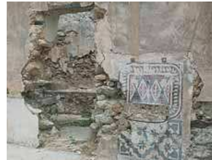
Close up of the main church of the Armenian Convent of St. Makarios in Chalefka showing the obvious signs of destruction.
