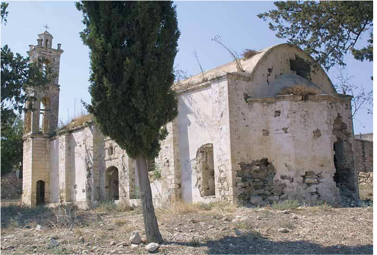
The church of St. George in Ardana clearly showing the signs of destruction.
