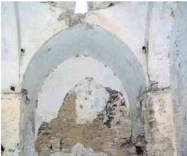
Only fragments of medieval frescoes remain on the west wall of the church.
